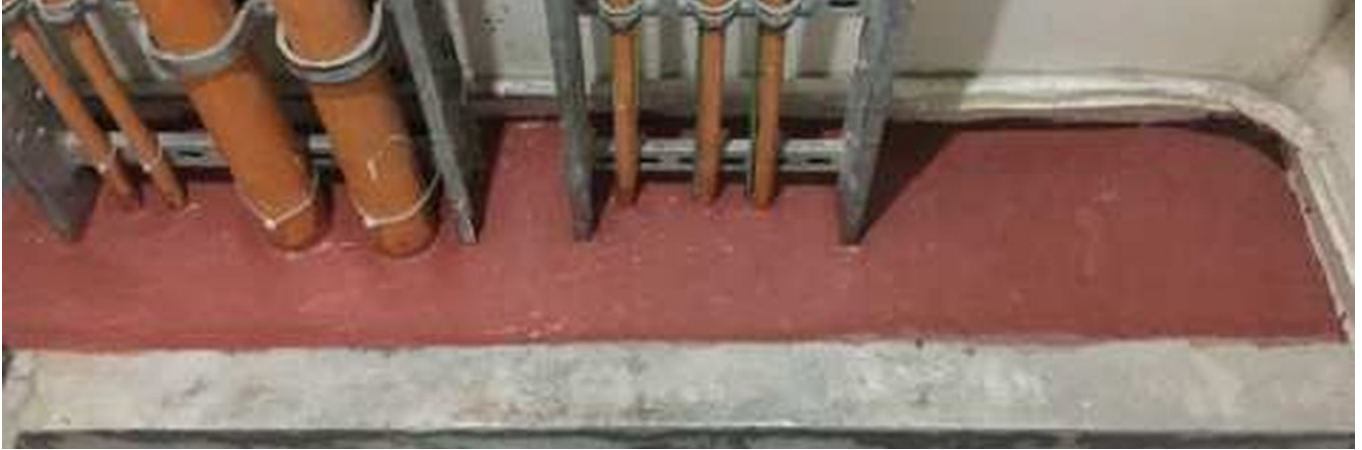
Multiple service penetrations through a floor
