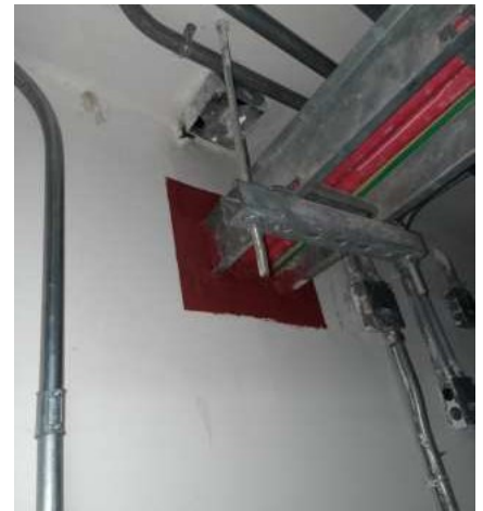
Cable tray penetration
