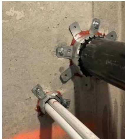
Pipe penetration collars
